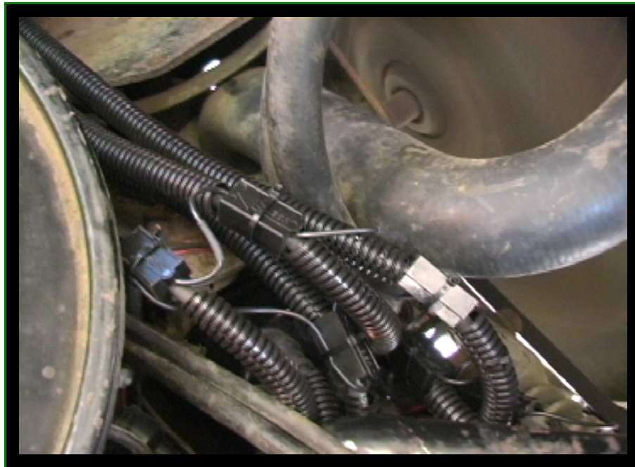
JPEG 2 - Ionizer Blocks installed on Champion 440 c.i. RV (seen during a road test). Note the "split loom" and the direct connecting wire layout.
